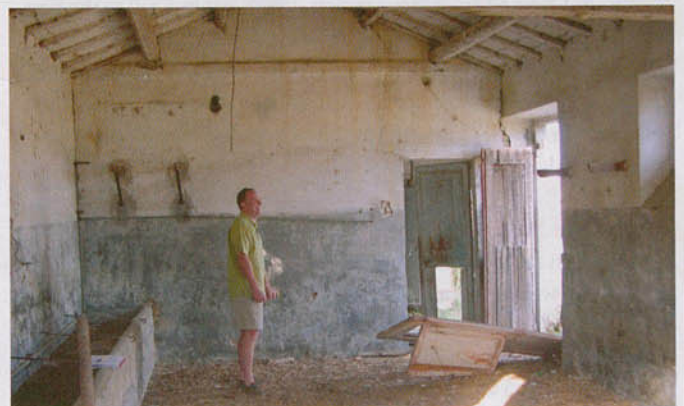
Left to right: The rear of the house; The pool was paid for with a redundancy settlement; Bob in house during renovation – this was to become a living room
